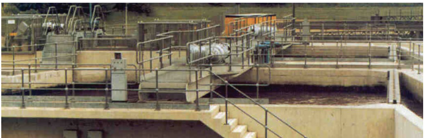
An installation of two 12.0m diameter Crossflow grit removal units.
